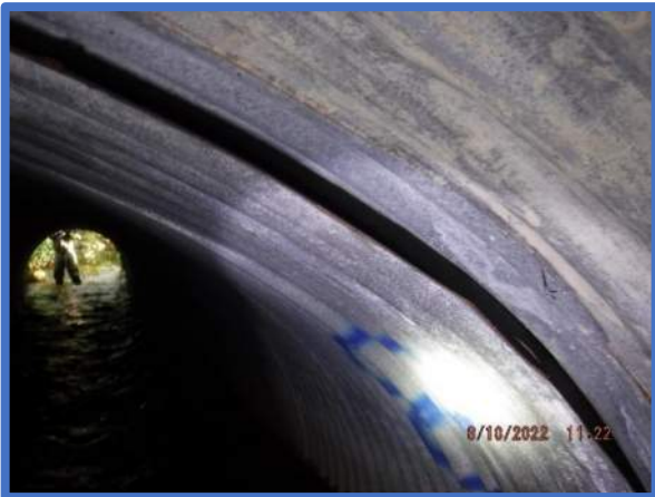
Image 3 – 2-inch gap at 33 feet
