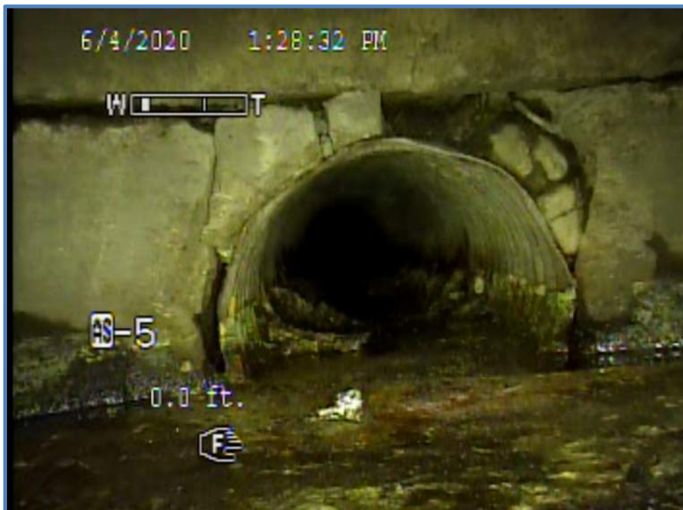
Photo 2 - Grout/Concrete failure at Pipe Penetration (MOA Pipe ID # 1538-26036)
