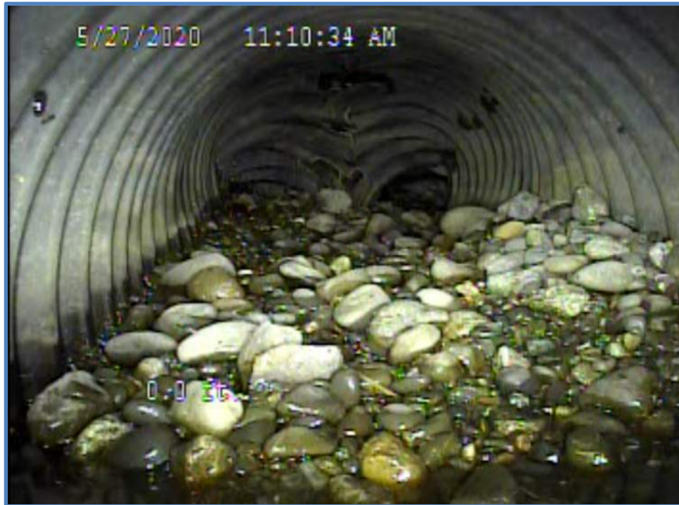
Photo 1 - Collapsed Pipe with Debris (MOA Pipe ID # 1538-32512)
