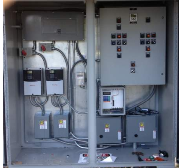
Photo 8 - Example Control Panel with VFDs Left Center
