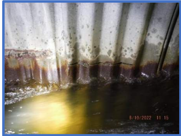
Image 2 – Cuts at 13 feet appear to be welded
