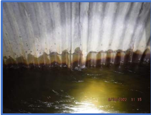
Image 1 – Cuts with surface corrosion at 13 Feet
