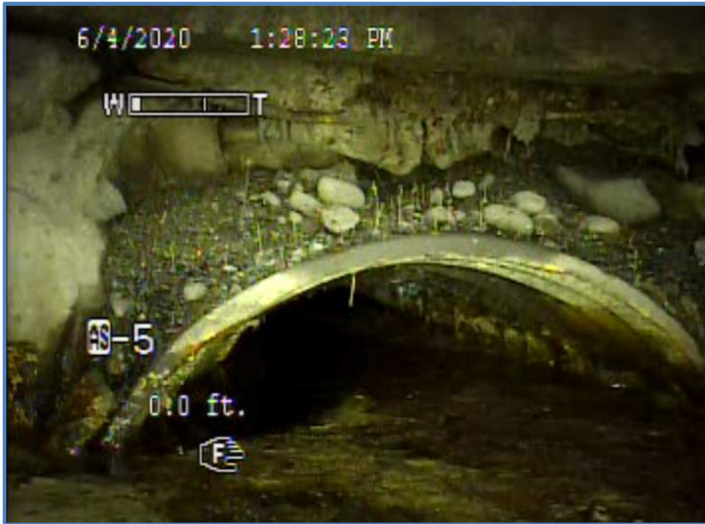
Photo 3 - Backwater from South Fork Chester Creek (MOA Pipe ID # 1538-24114)
