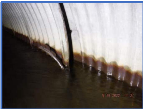
Image 5 – 4 Inch gap at 88 Feet pipe joint
