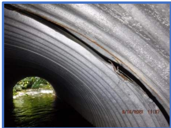
Image 6 – Beginning of gap at 88 Feet
