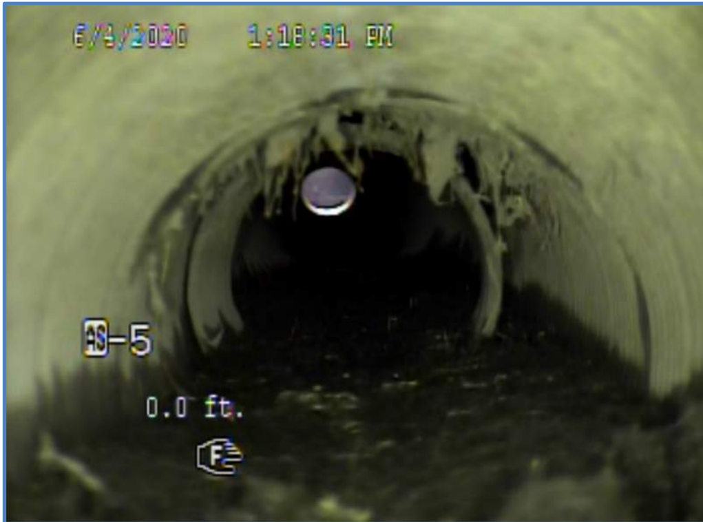
Photo 5 - Pipe Joint Separation & Debris (MOA Pipe ID # 1538-15612)
