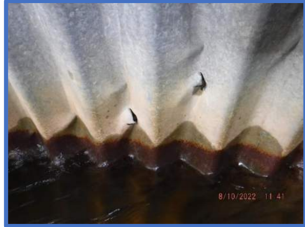
Image 8 – ½ inch diameter holes in pipe wall
